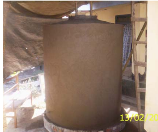
Ferro cement water storage tank at District Hospital Campus, Tamenglong
