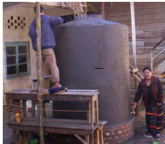
Ferro cement tank for storage of rain water installed at Ukhrul district
