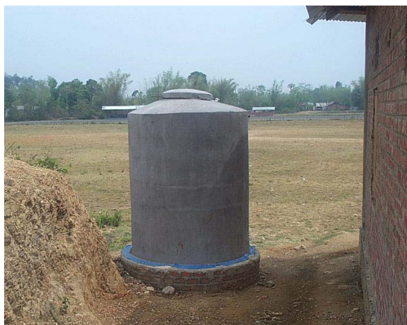
Ferro cement water storage tank at Langjing Achouba village, N.C. Road
