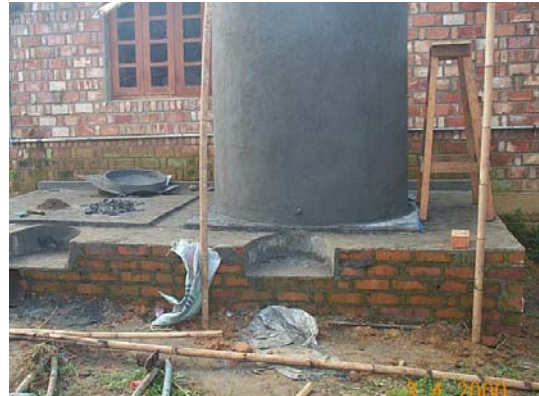
Base foundation made of bricks above which one tank was installed
