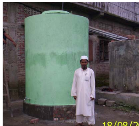
Rain water harvesting structure installed at Orphanage home
